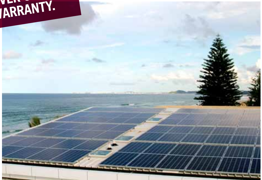
20.64 kWp system in Mermaid Beach, QLD
